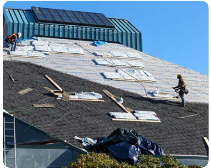
Roof work began in Fall 2023 and is expected to be complete this April.
